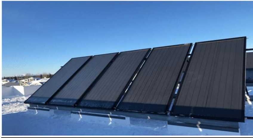
Figure 8: Flat Plate Solar Thermal Panels
